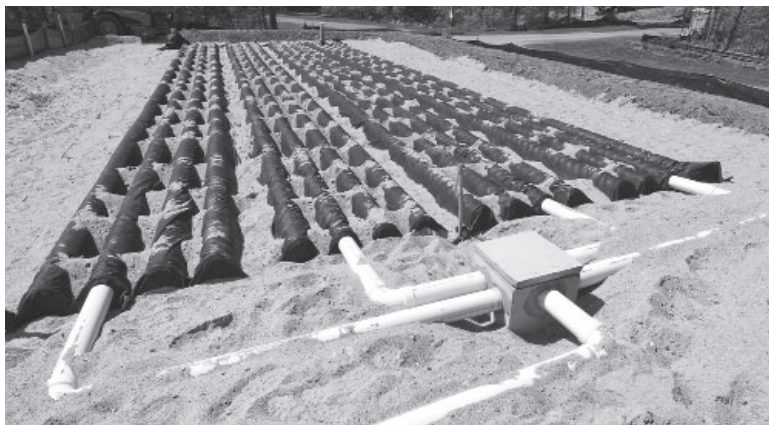
Septic system filter field installed in soil. This part of the septic system disposes of the septic tank effluent. The sewage effluent water is purified as it percolates through the soil.
